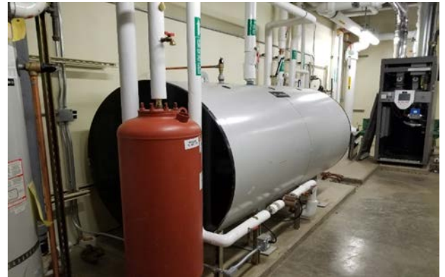
Boiler at Blackfeet Dormitory in Montana
