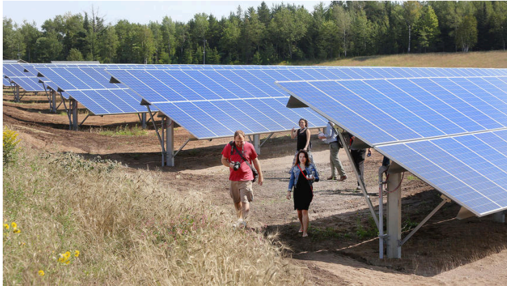
Community scale 1 MW solar array installed at the Fond du Lac Band in 2016
