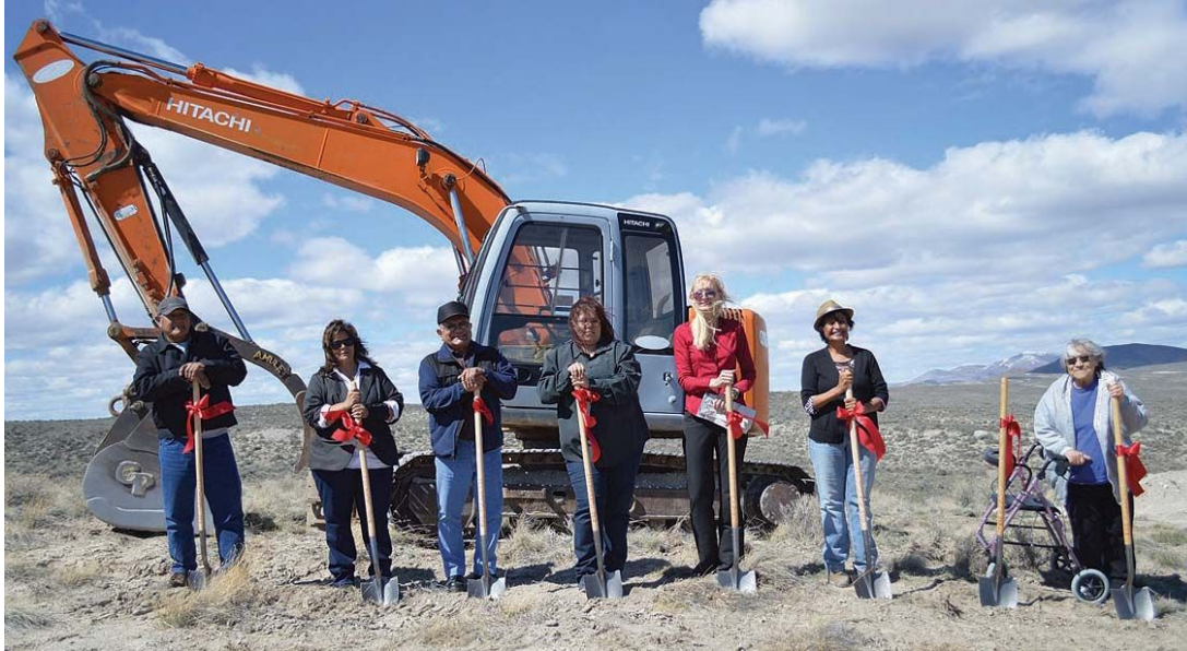
Wells Band business development center groundbreaking in April 2013. (Photo: Cindy Joyce, Elko Free Press).
