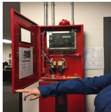
Testing the fire alarm system
