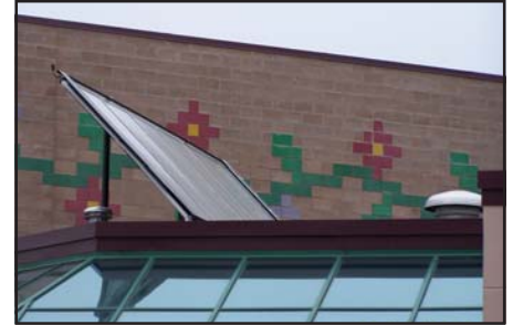
This solar panel heats water used in the gymnasium and cafeteria at Lac Courte Oreilles.
