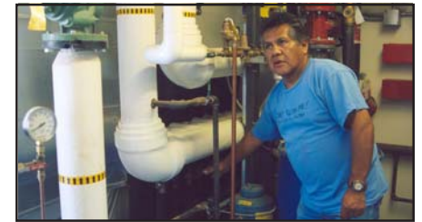
Seba Dalkai maintenance worker Larry Oso checks the school's geothermal heating pipes.
