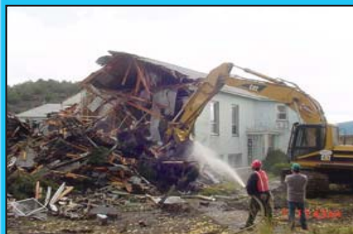
The Jicarilla Agency Building in Dulce, N.M., is demolished in October. The Agency offices are now housed in portable buildings.
