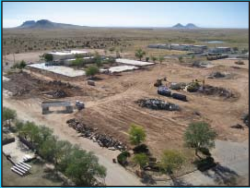
A phased demolition of old buildings will make way for the construction of the Dilcon Community School replacement campus north of Winslow, Ariz..
