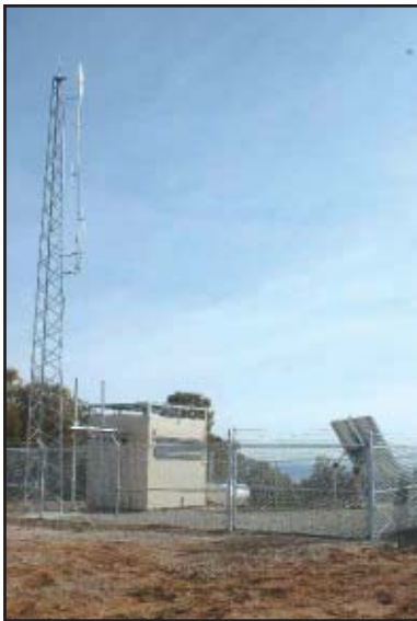
A renovated transmission tower site sits atop a mountain on the Acoma Pueblo Reservation in New Mexico.
