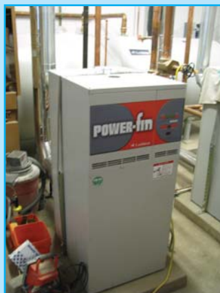
The heating units for inside air and for hot water are high efficiency and are connected to a computer-based building management system which will ensure their operation is reduced during off-peak hours.
