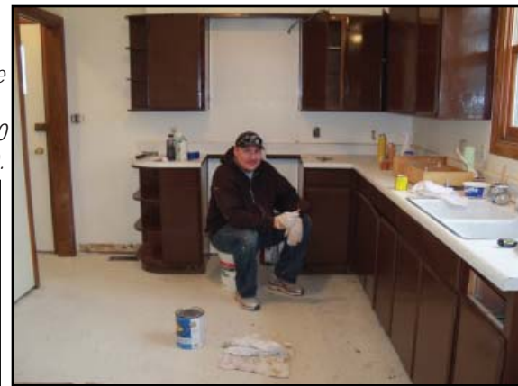
Hugh Traversie, a Cheyenne River Agency ARRA OJT worker, remodels the kitchen inside an employee quarters.
