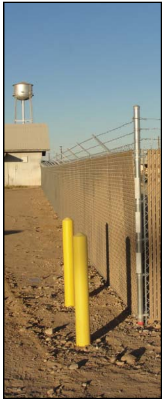
The facility management yard at the Colorado River Agency in Parker, Ariz., is enclosed by a new security fence.
