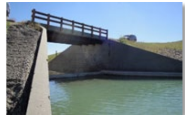
Willow Creek Dam and bridge over service spillway at the dam crest
